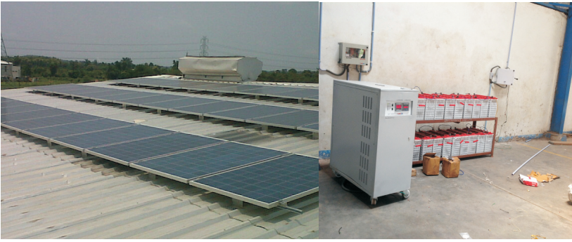
VRL Logistics Ltd, Gondkhairi, Nagpur 20 KVA / 240 V
