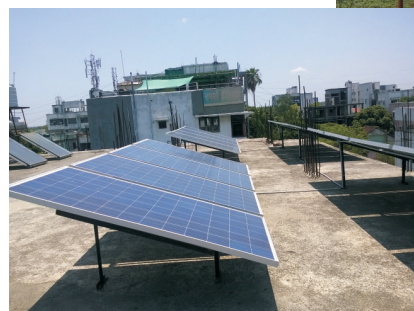
HP World Showroom Nagpur 4 KVA / 96 V
