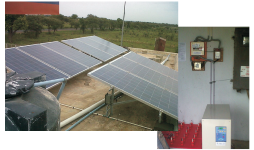
Mahindra Petroleum, Gadchandur Chandrapur ; 5 KVA / 72 V
